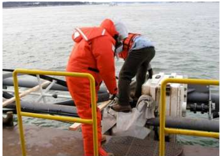
Bob Lewis (left), ORPC's general manager, and contractor Steve Cox of Woodland Machine Works in Baileyville work on development of ORPC's prototype off Eastport in December 2007.
